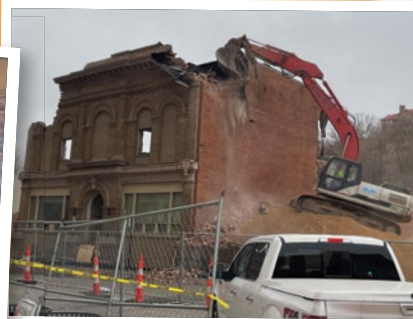
The historic former Knights of Columbus Hall in downtown Dubuque came down last week to make way for a new childcare center to serve employees of Cottingham & Butler as well as other downtown workers.
